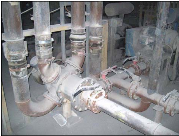
Air Pipework Manifold to Homogenizer
